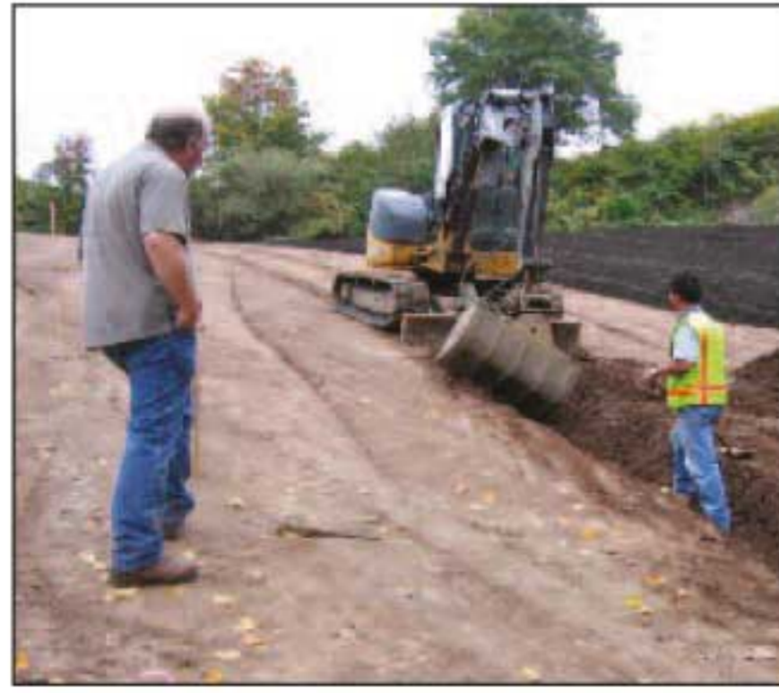
A light-duty backhoe is all that is needed to dig the shallow trench in preparation for the SmartDitch installation.
