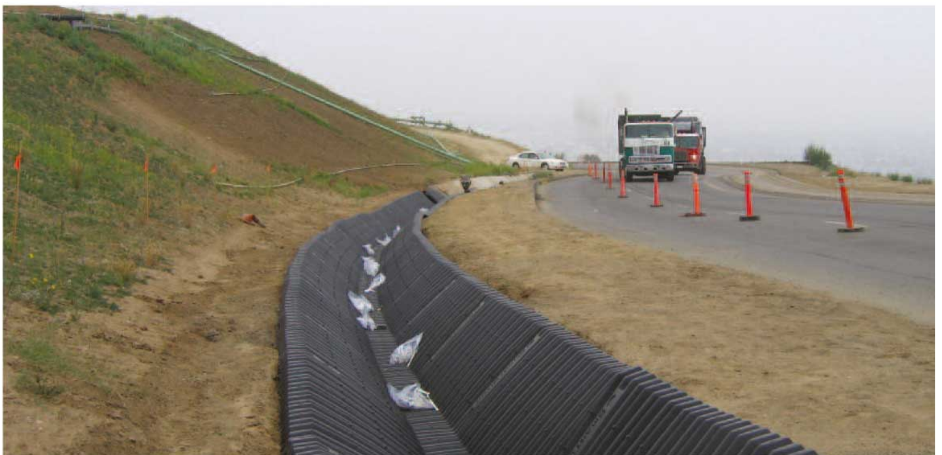
Initially, SmartDitch was installed in a channel at this Puente Hills Landfill site to temporarily control a conveyance ditch. However, considerable settlement over time made the use of concrete channels (originally specified) unusable and SmartDitch became the permanent solution.
