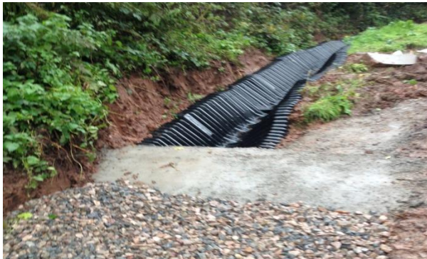
The SmartDitch flows into a culvert at a passing place
